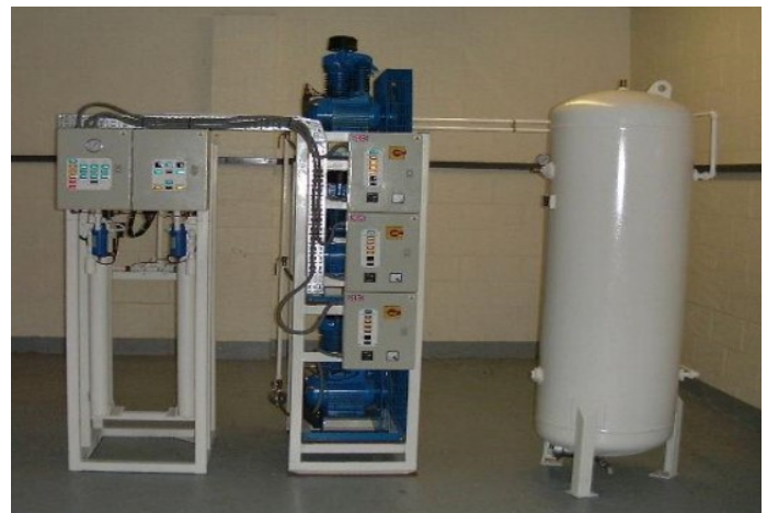
Triplex Medical Air Plant
