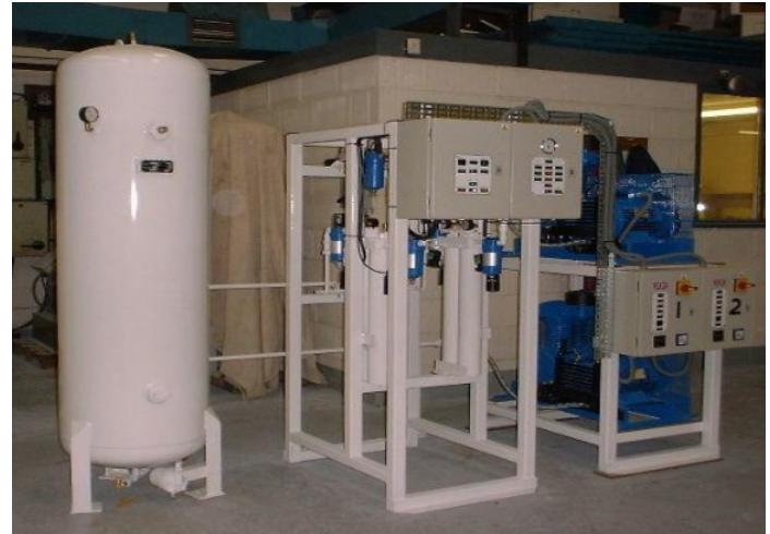
Duplex Medical Air Plant
